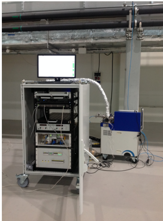
Figure 1: The SOLARIS Heating Unit Controller.
