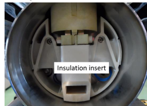
Figure 5: Insulation insert installed, covering the bare bus-bars and protecting the diode venting channel.
