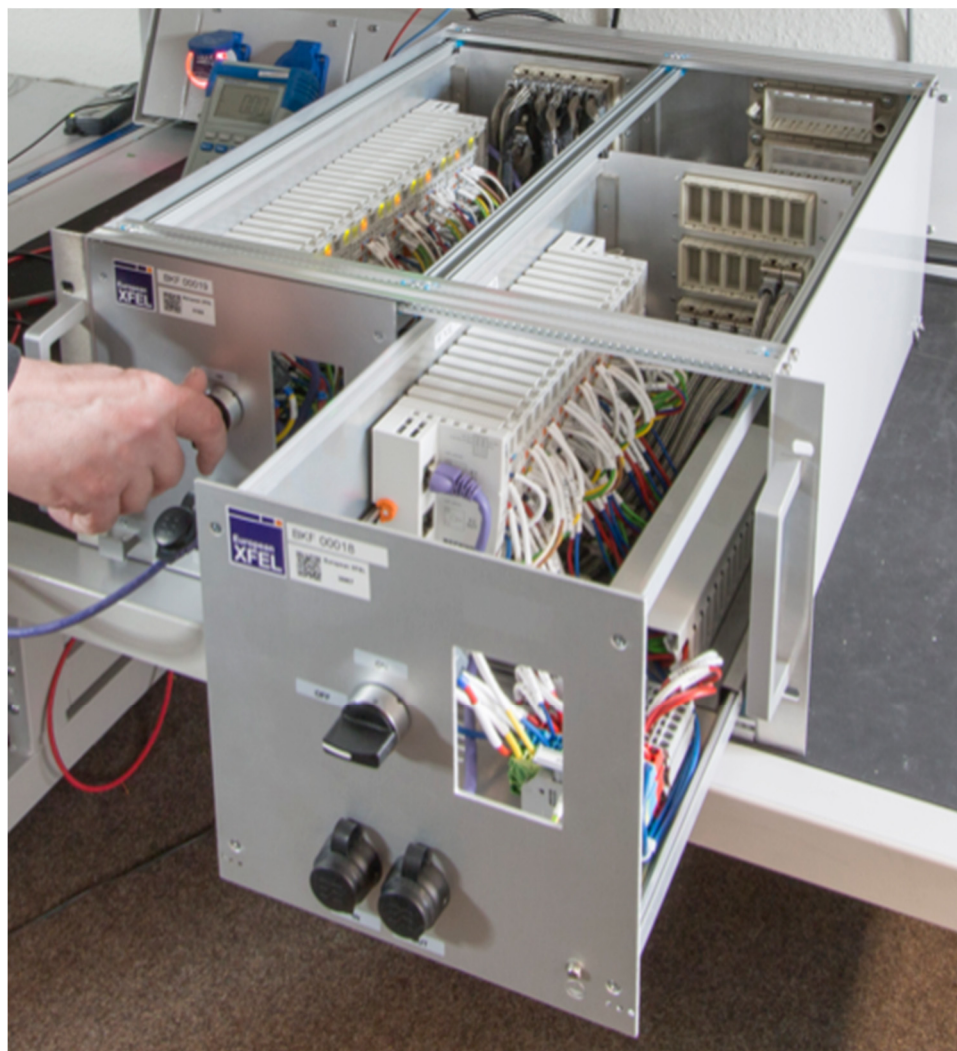
2 PLC modules in one 19" frame
