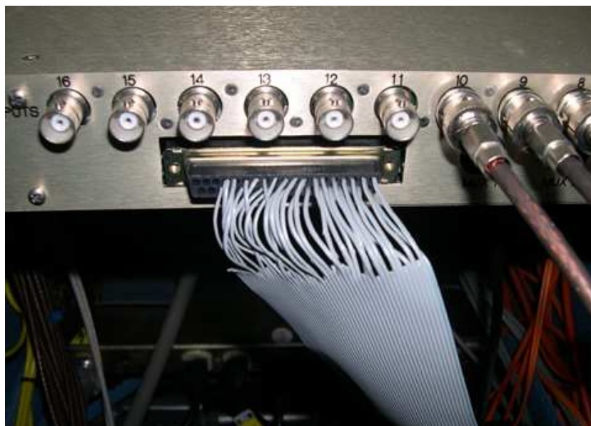
Figure 2a. An example of a signal concentrator ribbon cable. Detailed conductor-by-conductor information is required for this situation.
