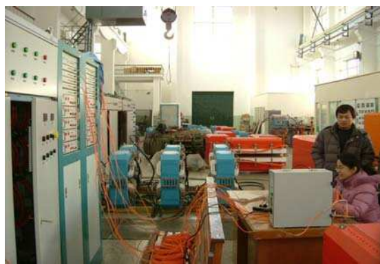
Figure 8: Chopper PS Control Testing on-site
