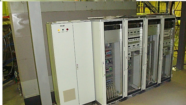
Power supplies of injection
