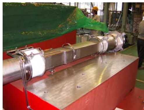
Figure 6: Collimator duct is fixed on the shield block.
