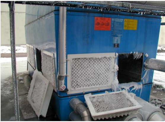
Figure 2: Cooling tower with ice up intake openings
