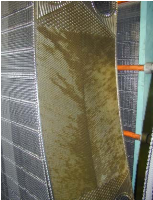
Figure 3: Dirty heat exchanger plate
