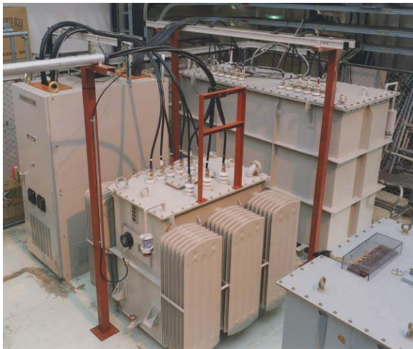
Figure 2: New klystron power supply as installed.
