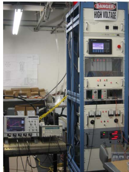
Figure 2: Charging power supply rack picture.
