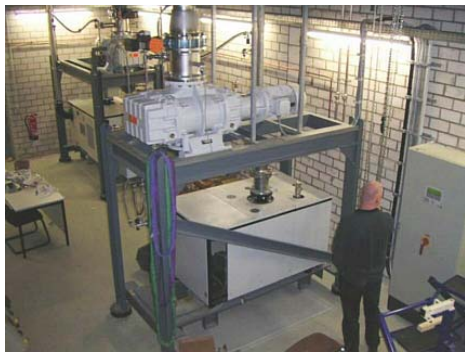
Figure 2: A combination of Leybold RA7001FU roots blowers and Sogevac SV1200 rotary vane pump is used to pump the HOBICAT helium bath to 16 mbar.
