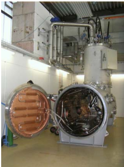
Figure 1: The HOBICAT cryostat and feedbox in the radiation enclosure.
