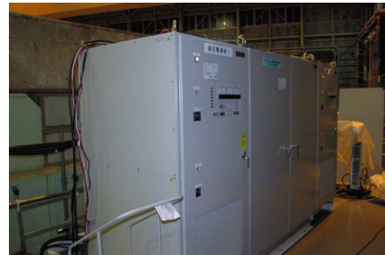
Figure 8: Power supply of kicker magnet
