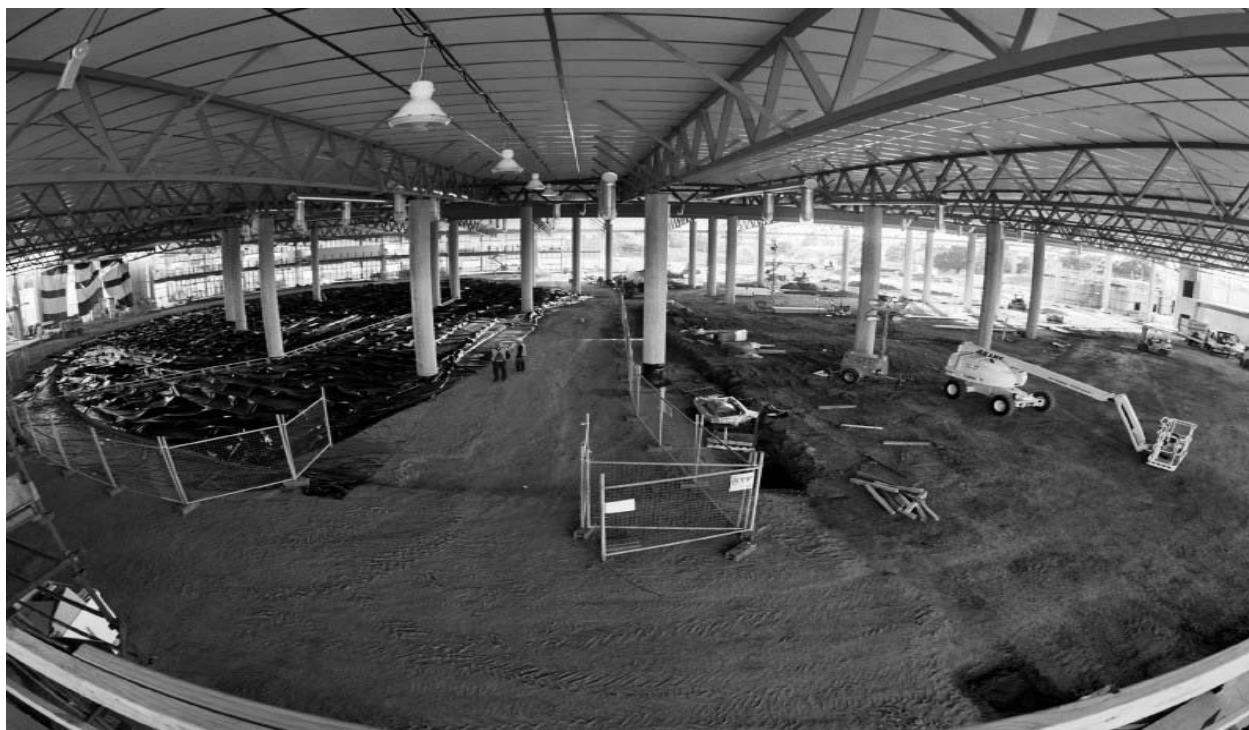
Figure 3. A view of the interior of the facility taken from the mezzanine floor (June 2004).
