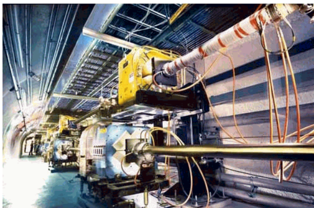
Figure 1 View of the PEP-II tunnel.
