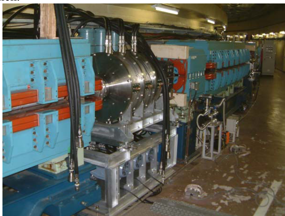
Figure 1: A set of installed induction cavities in the KEK-PS
