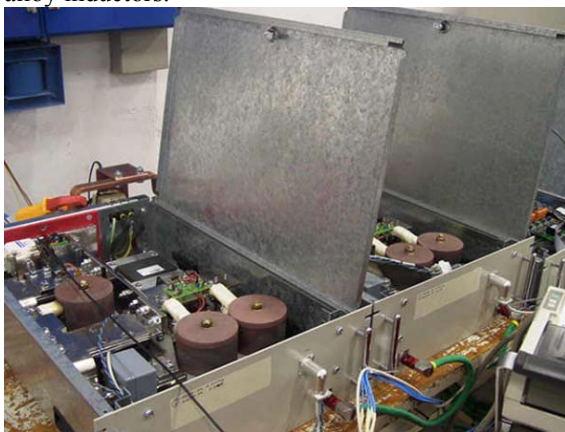
Figure 2: Sub-converter 8V, 2kA output module
