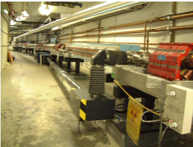
Figure 1: Location 1C12 in the Hall A beam line with the installed synchrotron light interferometer.
