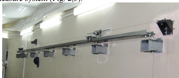
Figure 2: Installed survey wall targets with adjusted distance measure system.
