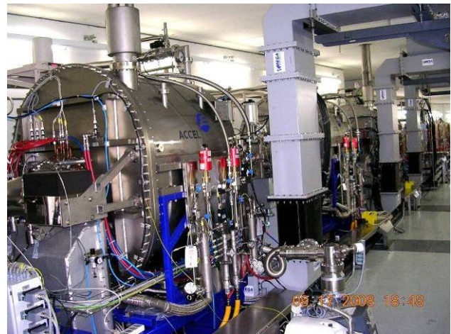
Figure 1: SRF modules in the tunnel of storage ring
