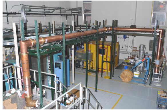
Figure 3: Test facility showing FPA test platform on left, capacitor bank in middle, water load/circulator on right
