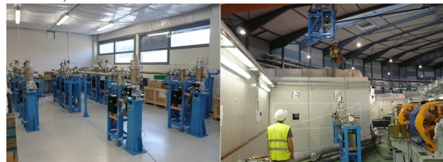
Figure 6: the assembly of the front end in the lab. and during the installation in the tunnel.
