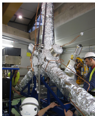
Figure 5: the RF cavity of the storage ring during the installation inside the tunnel.
