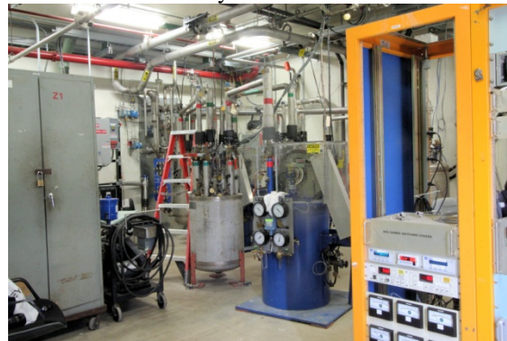
Figure 3: MTA Refrigerator room
