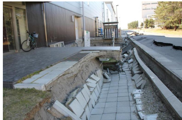
Figure 1: The entrance to the linac building, where a footpath subsided.
