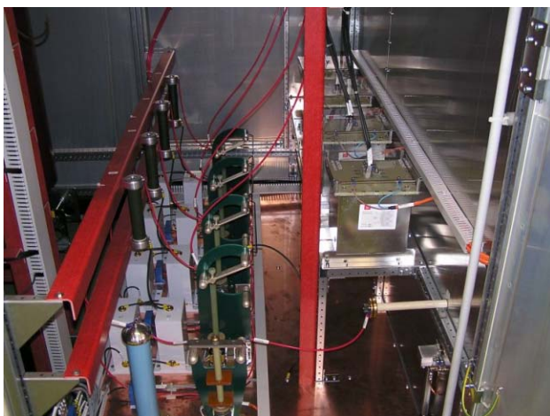
Figure 3: High Voltage Distribution
