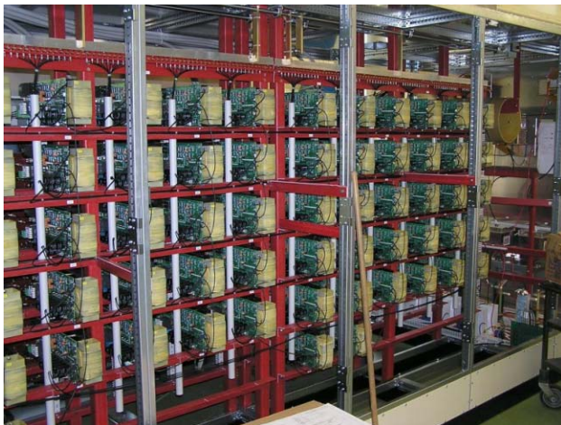
Figure 2: Power Supply Unit
