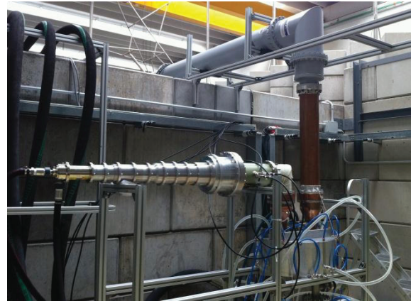
Figure 4: Detail of the High Power Coupler test Stand. Coaxial waveguides, the coupling cavity and the water load are recognizable.
